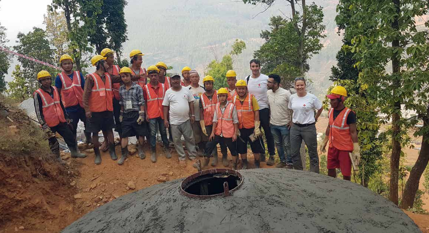
Construction supervision of reservoir tanks in rural Nepal, Austrian Red Cross with Nepal Red Cross, May/June 2019
